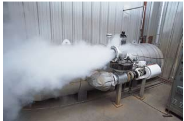
Following repair, a specially designed steam boiler assists with testing of pressure relief valves.
